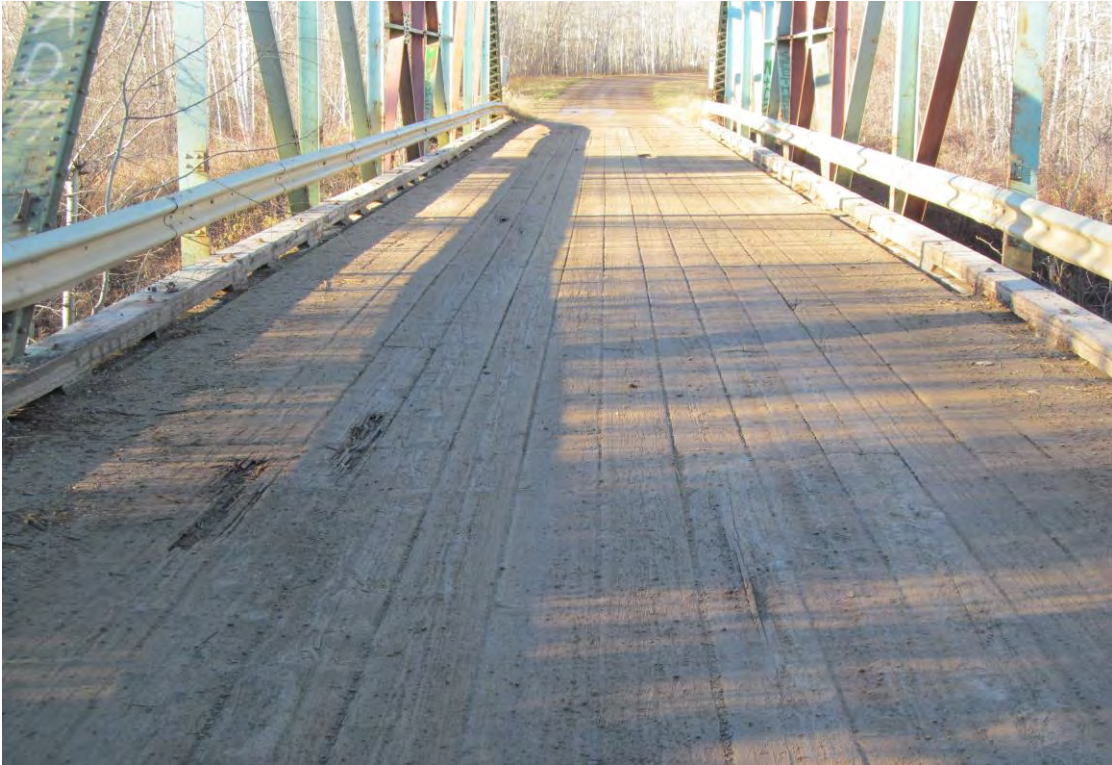
Photo 1 Typical strip deck condition, should be replaced soon
