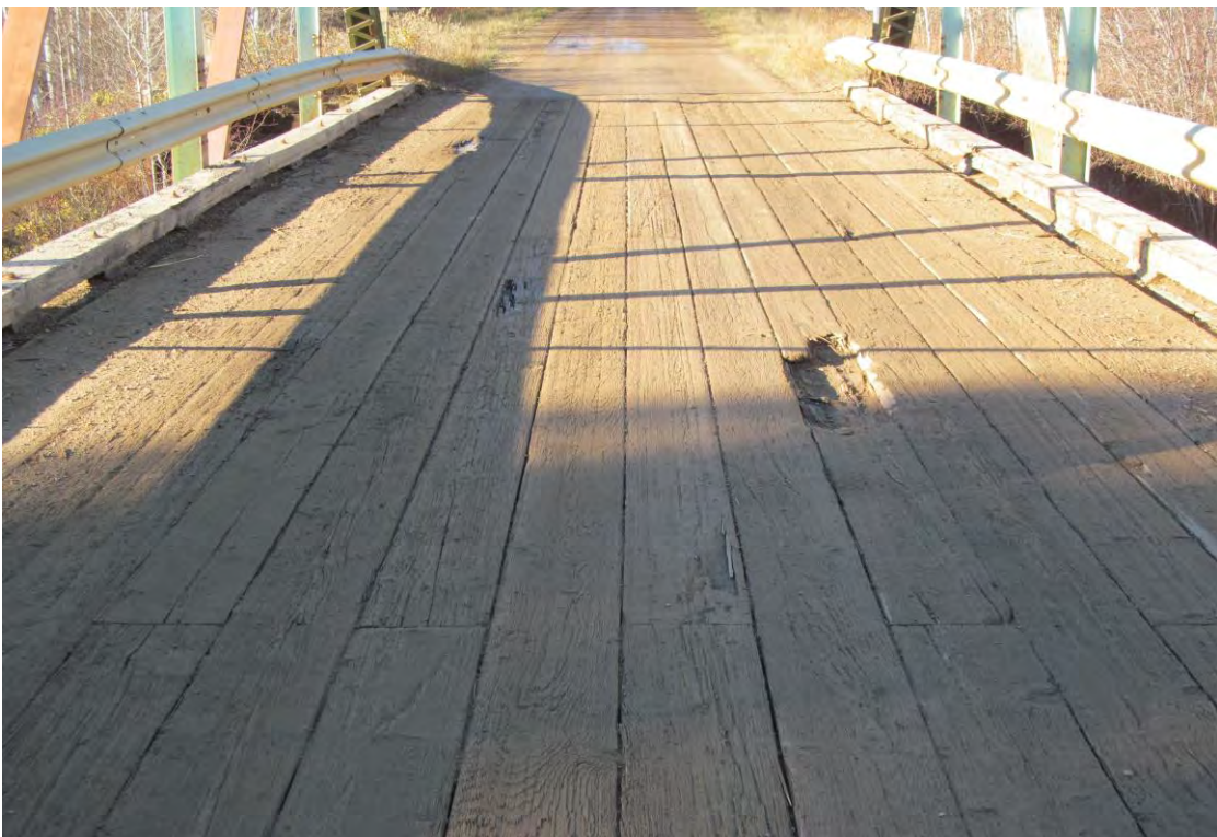
Photo 2 Close up of the strip deck, some planks have pot holes
